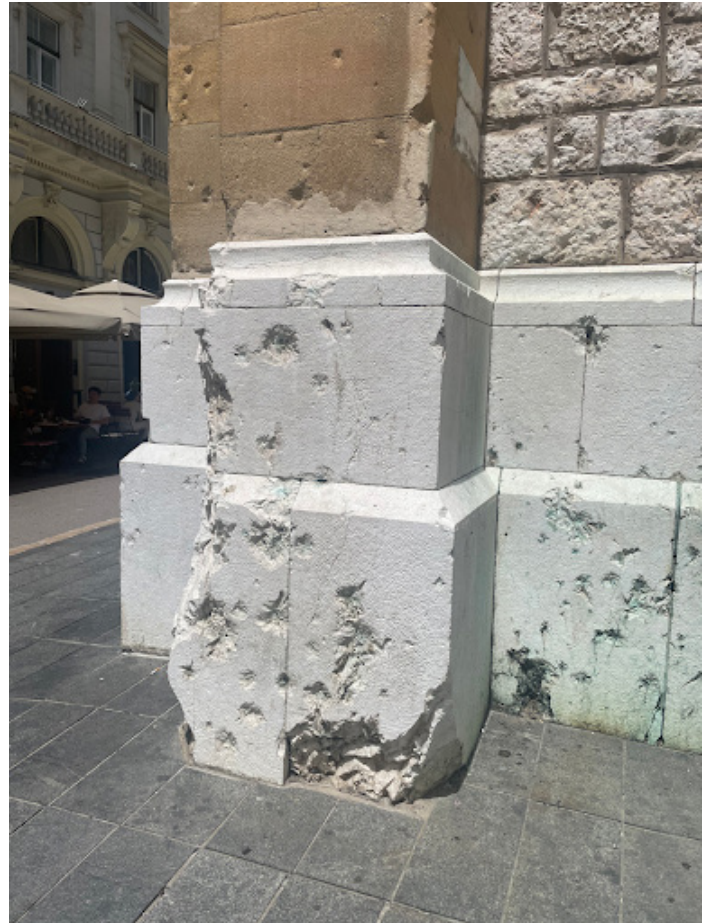
Figure 2: The Sacred Heart Cathedral in Sarajevo’s city center. While much of the building’s war damage has been repaired, bullet holes still chip away the cornerstone. Photograph taken by Evan Daneker.
