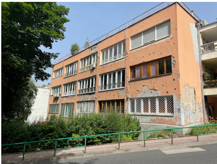
Figure 3: Bullet holes pierce the facade of an apartment building in the Mejtas neighborhood of Sarajevo. Photograph taken by Evan Daneker.
